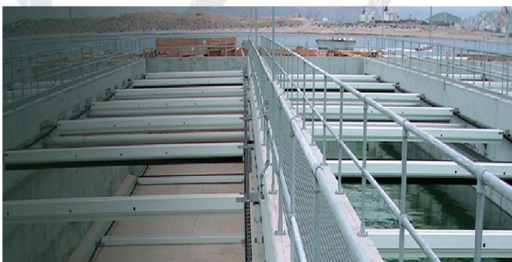
Scraper & skimming mechanism for Rectangular Clarifier basin
