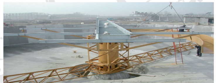
Clariflocculator with twin scraper arms & central driven torque tube
