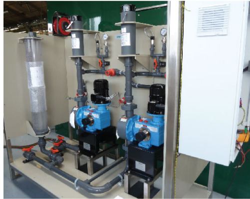
Chemical Dosing System
