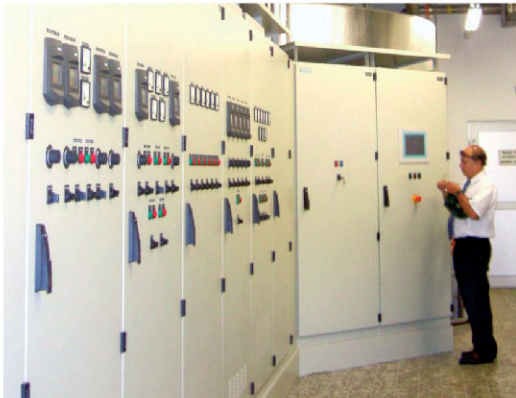
Motor Control Center
